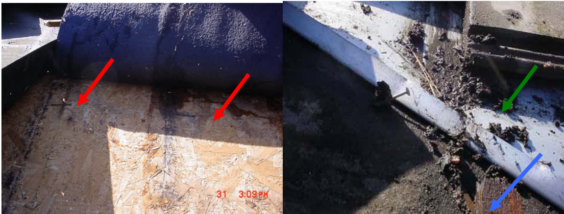
Figure 13. Image (left) showing the underlayment and roof sheathing, as well as two nails (red arrows) found lying on the roof sheathing. The heads of the nails penetrated the underlayment, causing water to flow onto the roof sheathing and then into the residence. The image on the right shows remains of the debris dam and the edge of the flashing (green arrow) where the water spilled over (blue arrow).
