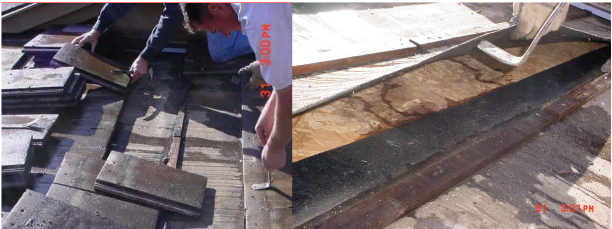
Figure 12. Images showing water under the tiles (left) and under the roof's underlayment (right). Note the location of the area in reference to the gutter at the upper left side of the left image.
