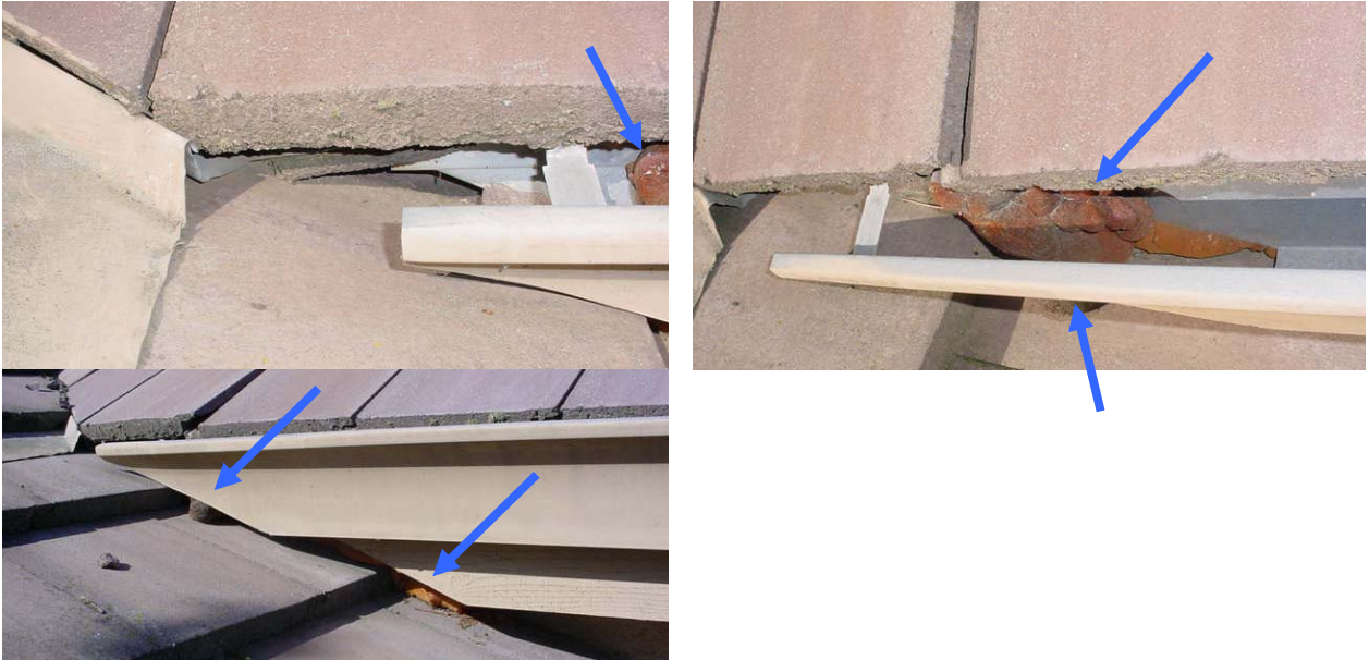
Figure 4. Visual images showing a close-up of the gutter system (Fig. 3) where foam was applied. The foamed area (blue arrows) may be covering a possible water intrusion point.
