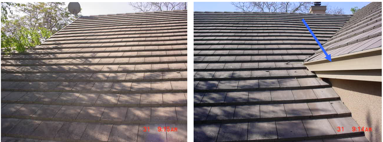
Figure 3. Visual images of the roof showing the cement roofing tiles intact (without cracking, separation or missing tiles). The gutter system at the right (see blue arrow) did have unusual construction, as shown in Figure 4.
