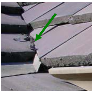
Figure 14. Image showing the debris dam at the roof valley before the tile was removed.
