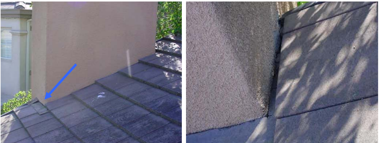
Figure 5. No flashing is visible at the chimney's top and side but may be incorporated within the chimney's cladding, which is stucco. This is apparent in the visible flashing of the chimney's lower edge, as shown on the image at the left (see blue arrow).
