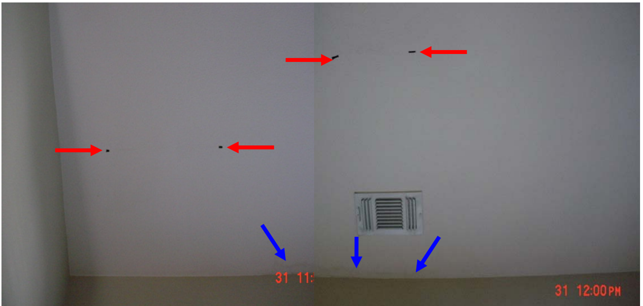
Figure 2. Visual image of the living room ceiling showing the water staining caused by the roof leak. The blue arrows show the staining along the ceiling-wall joint directly under the supply register. Black marks (pieces of tape indicated by red arrows) are reference points for the wallboard separation, only visible upon close examination between the tape marks.
