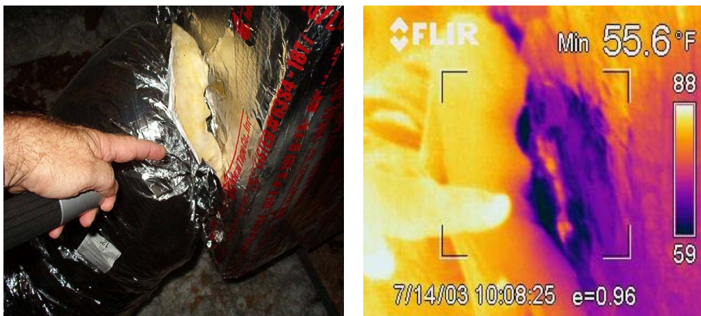
Figure 8. Supply junction of flex duct and disbursement box that was not sealed or taped
