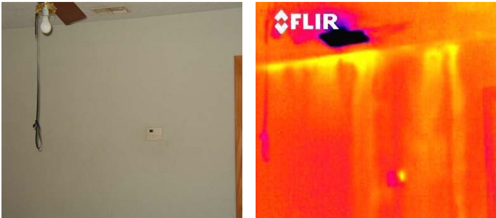
Figure 4. Thermal ducting inside a hollow wall behind the thermostat
