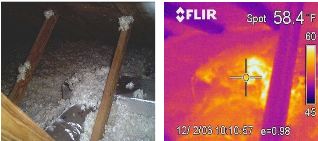
Figure 9. Supply leak showing heat loss under blown-in insulation
