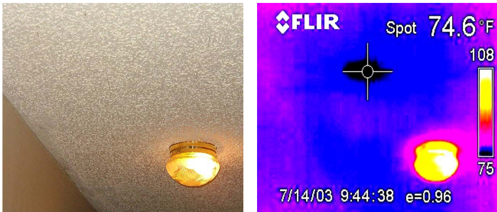
Figure 7. Cold spot on hall ceiling caused by supply junction leak in attic over ceiling board
