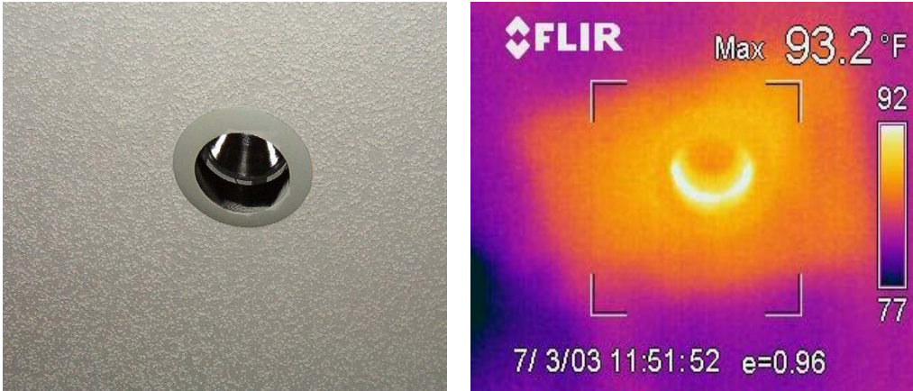
Figure 3. Ceiling penetration and insulation problem
