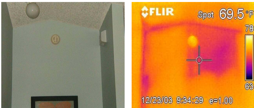
Figure 2. Areas of heat loss through a standing wall that is not insulated
